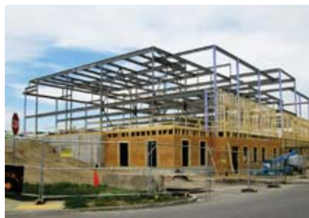
Under construction photo taken May 18, 2017 screening, and pharmacy will also be included for better patient care.”
