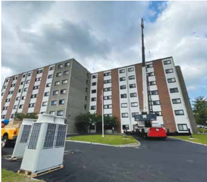
Crane lifting units to the rooftop. (Dana Nute, President of Resilient Buildings Group)
